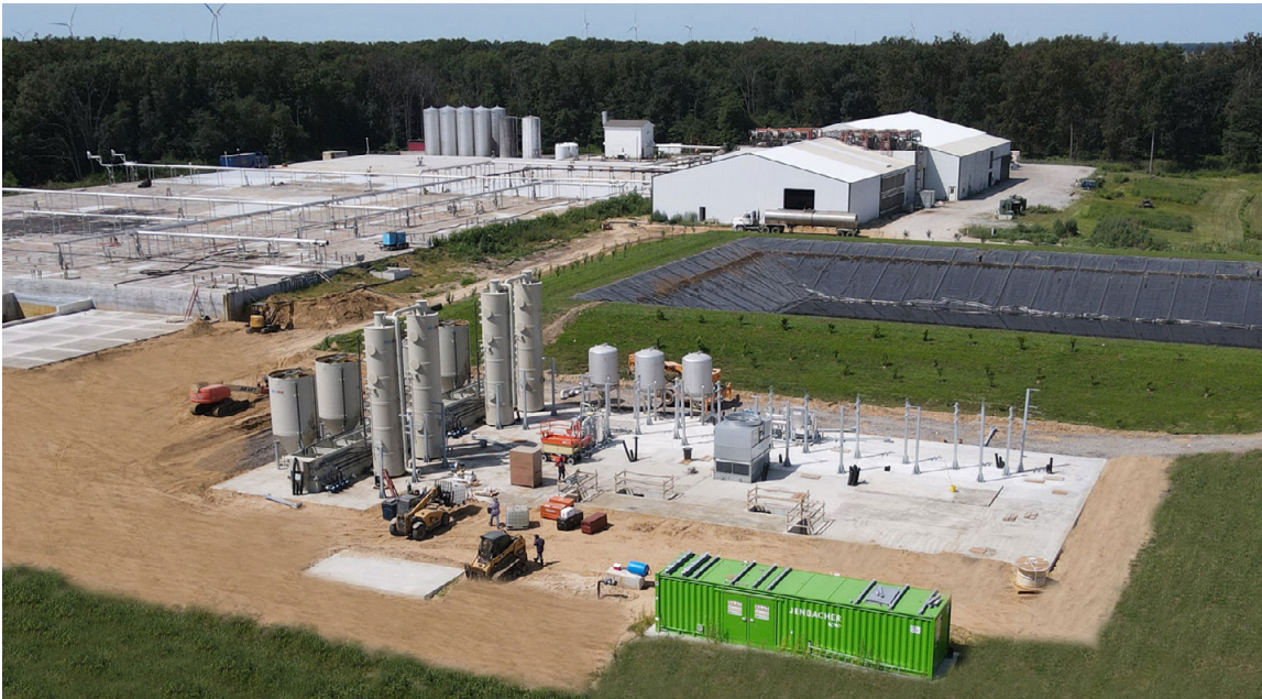
BioTown Biogas is headquartered in Reynolds, Indiana. (photo courtesy of BioTown Biogas)
